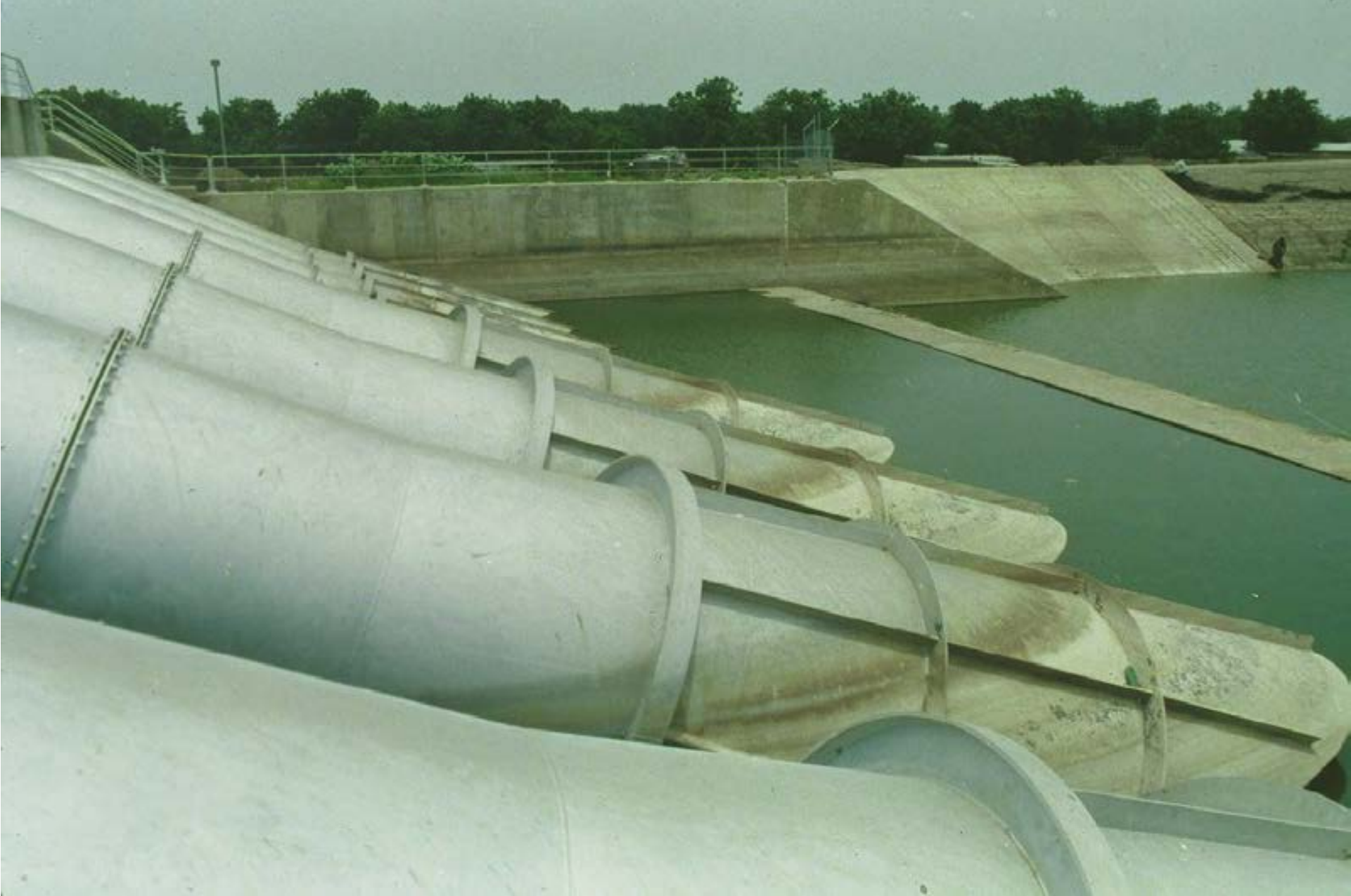
Photo 52: Faga pumping station, South Lake Chad Irrigation, August 1986
