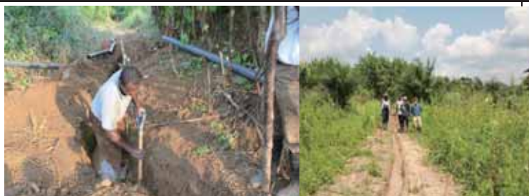
Restoration measure to connect spring water and sawah by irrigation canal and syphon pipes at Adugyama, Mr. Tawiah's site, August 2011
