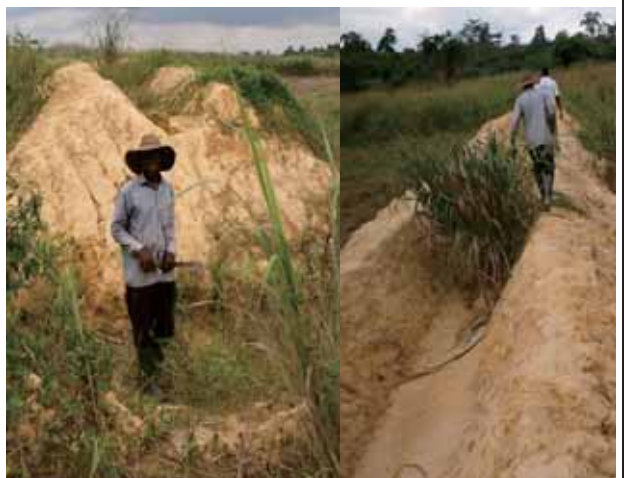
Fake irrigation canals, which is developed on upland higher than 2m from Biemo river. It is impossible to introduce water to the canal. Biemo No.1. Upper area of the dam completed, 2nd of September 2016
